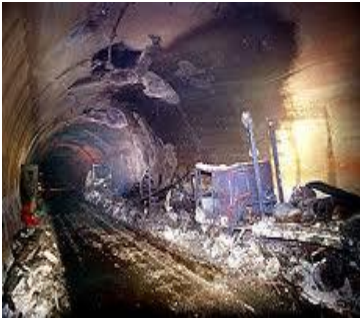
Fire spalled concrete
