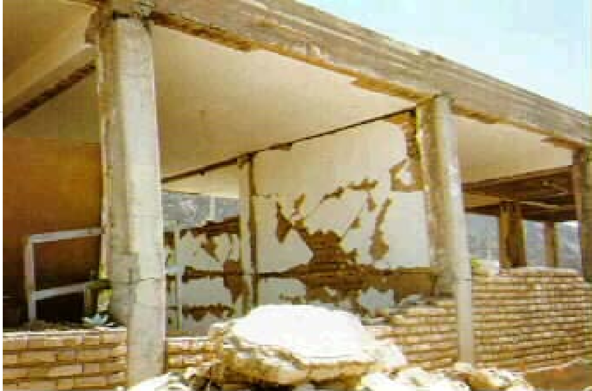
Ardekul 1997: Collapse of the upper part of the infilled walls in this reinforced concrete building created a short column effect. (Photo from CEST Report)
