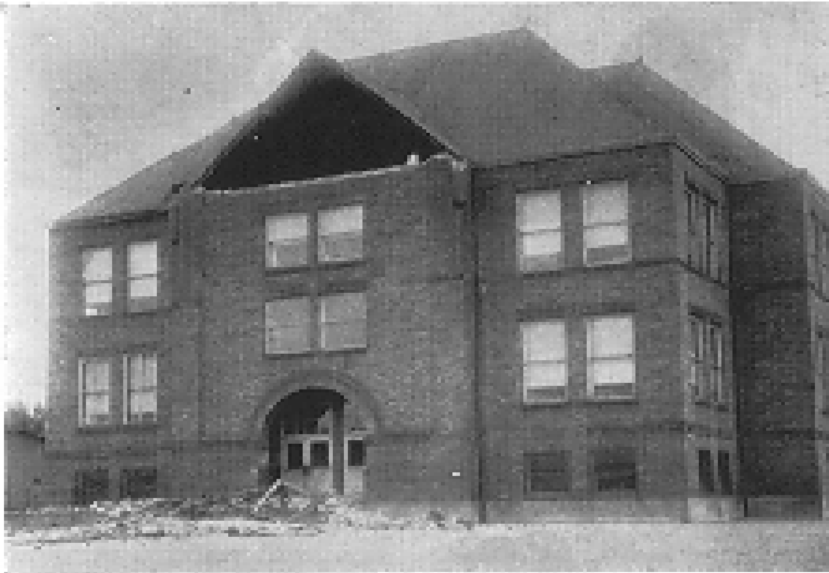
Lafayette School in Seattle after the 1949 earthquake. The gable fell because of lack of adequate anchorage and defective masonry. The masonry fell on the landing in front of the main entrance. (Photo from an article by C. N. Dirlam reproduced in Thorsen, 1986)
