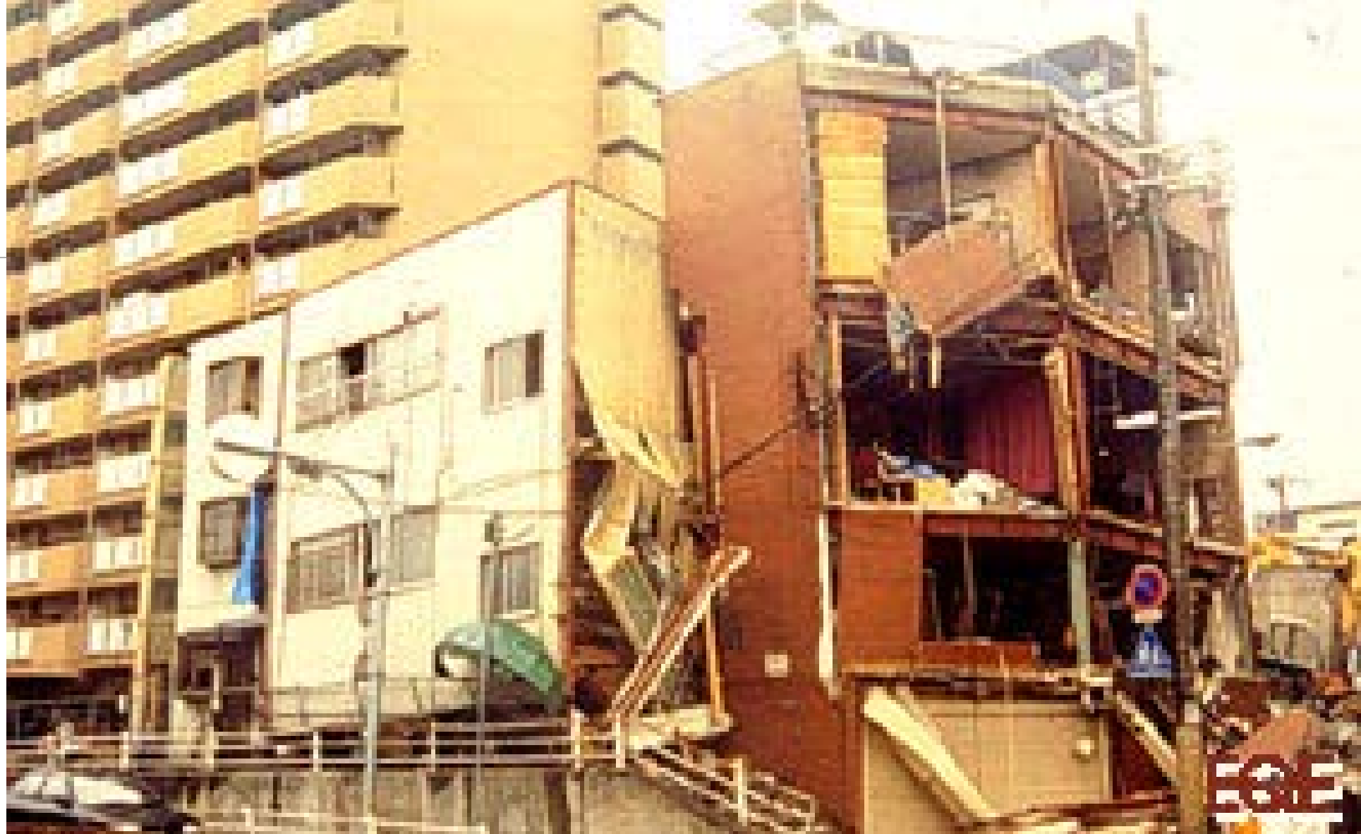
Kobe (1995): Steel buildings in the Nagata Ward. While the frames appear to be in good shape, the cladding was shaken off the building, posing a severe life-safety hazard
