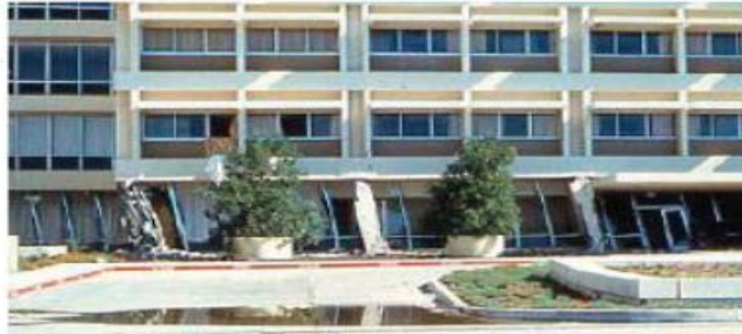
Figure 5-15: Olive View hospital, San Fernando earthquake, 1971, showing the extreme deformation of the columns above the plaza level.
