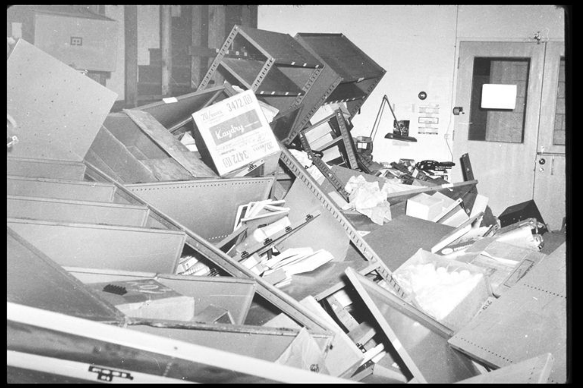
San Fernando, California earthquake, Feb. 9, 1971, Magnitude: 6.5 Damage to shelving and contents, Spectrolab 12484 Gladstone, Arroyo Light Industrial Tract
